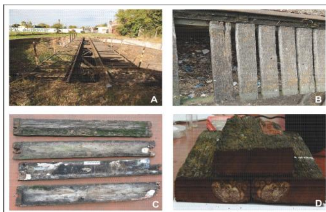
Fig. 2. Detail of locomotive turntable status: A - Structure consists in wooden slats of Schinopsis sp. within metal framework; B - slats in advanced status of deterioration caused by environmental and biological factors; C - Samples acquired for simulating the same degradation status than wooden turntable in laboratory; D - Detail of wood decay fungi found and its biodegradation (inside view).
